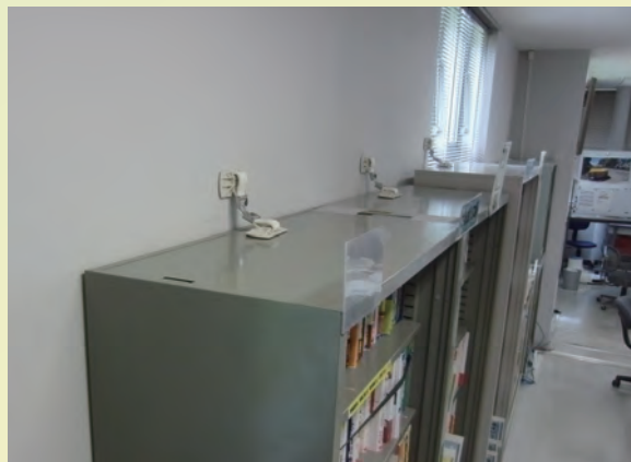
< Measures to prevent shelves from falling over >
